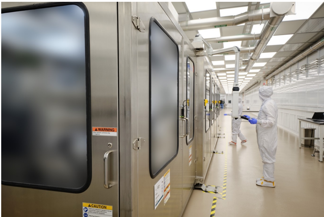
Separator processing equipment undergoing qualification.
